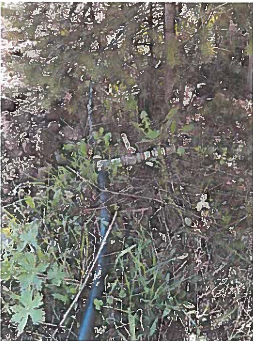
Photograph 6: Exposed water line on Balsam
