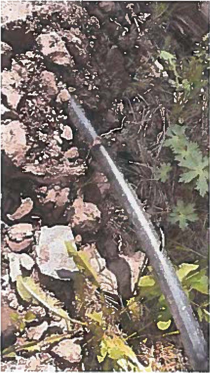
Photograph 8: Exposed water line on Balsam
