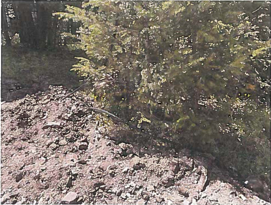
Photograph 7: Exposed water line on Balsam
