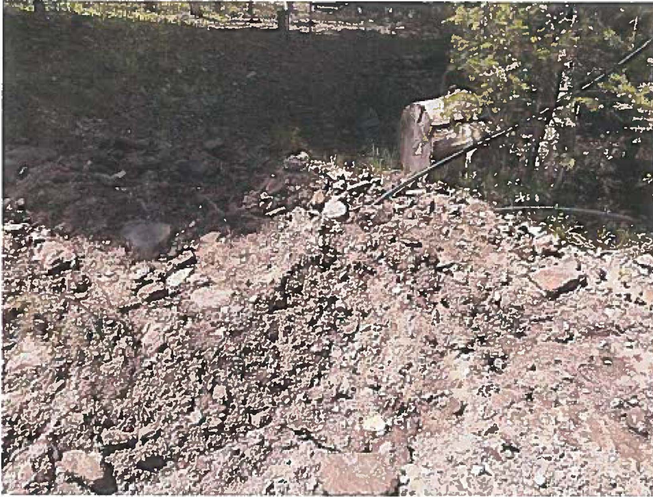
Photograph 5: Exposed water line on Balsam
