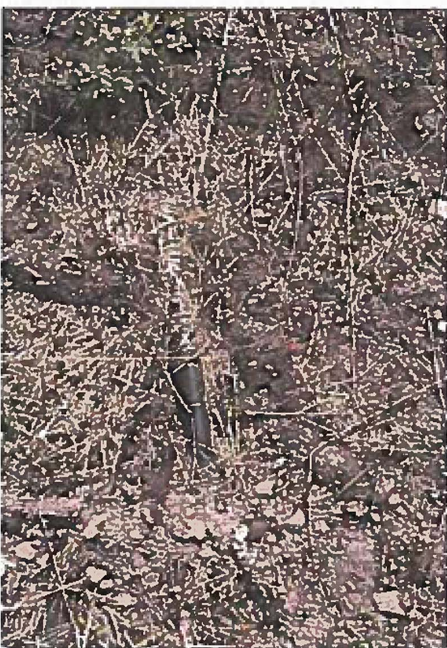
Photograph 4: Exposed water line on Balsam
